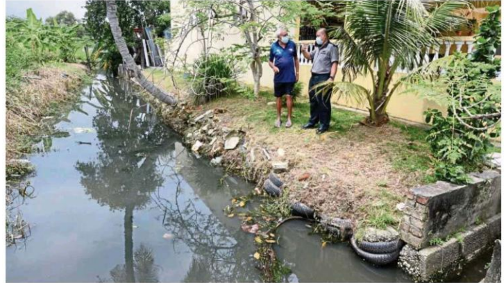
Azman (right) explaining to resident Serjeet Singh that the land status needs to be determined before the concrete drain behind the houses can be rebuilt.
